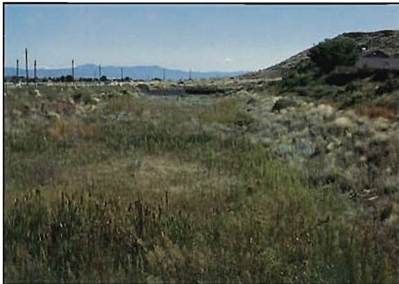
San Antonio Channel used a man-made mat to prevent erosion and to promote vegetation. Two years after construction, there is lush growth.
