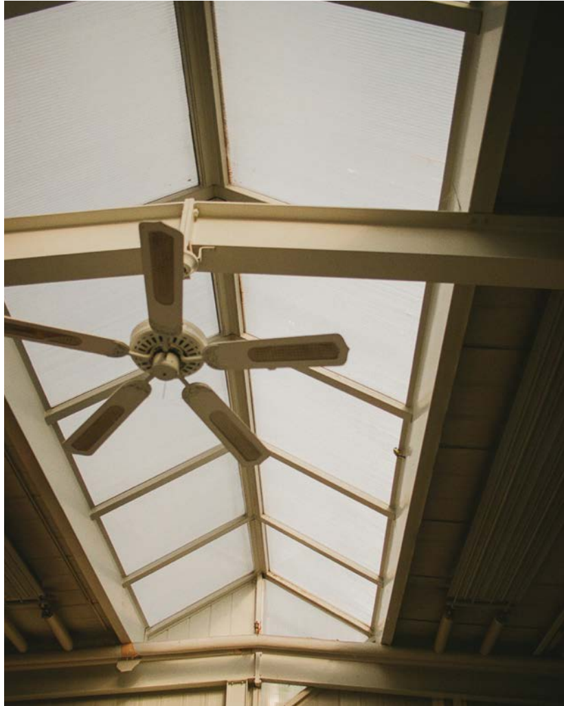
SHOWROOM HALL BROKEN VENTILATION ANALOG FOTO 12.2023
