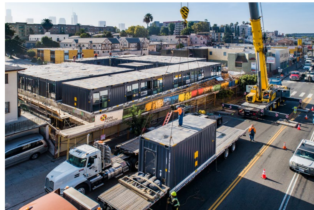
The steel modules for Hope on Alvarado were trucked to the site before being craned into place over a site-built concrete podium—a process that took one month to complete.
