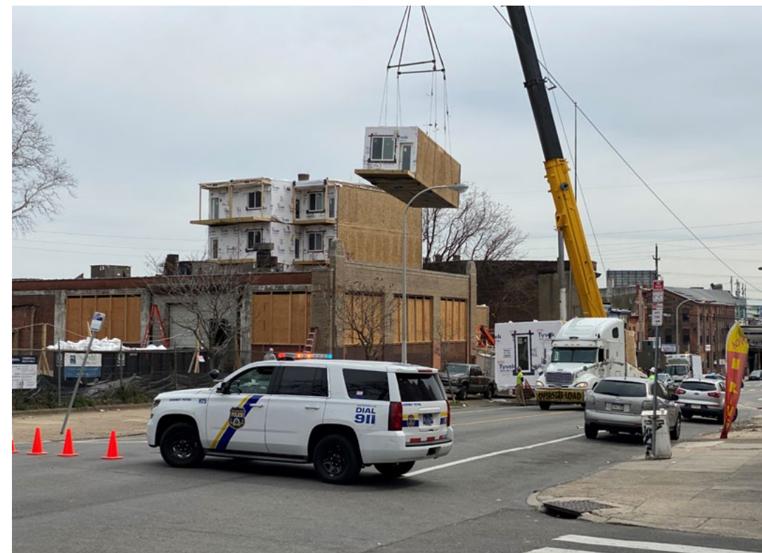
One of the 35 modular units is craned in at Golaski Lab Flats in Germantown, Philadelphia.
