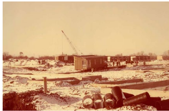
Modular construction was used to construct 295 units of housing in Indianapolis, Indiana.
