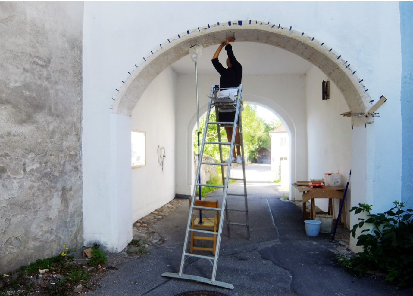
Detail of the process to make the replica of the arch of Taubenturm
