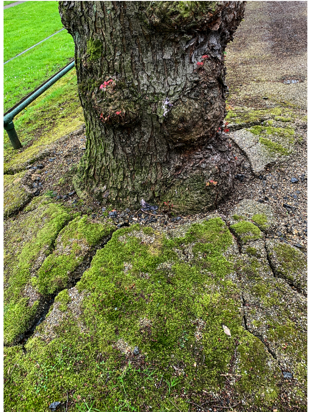
Figure 28: Captured in Rotterdam Noord, 2024: Tree cracking concrete.
