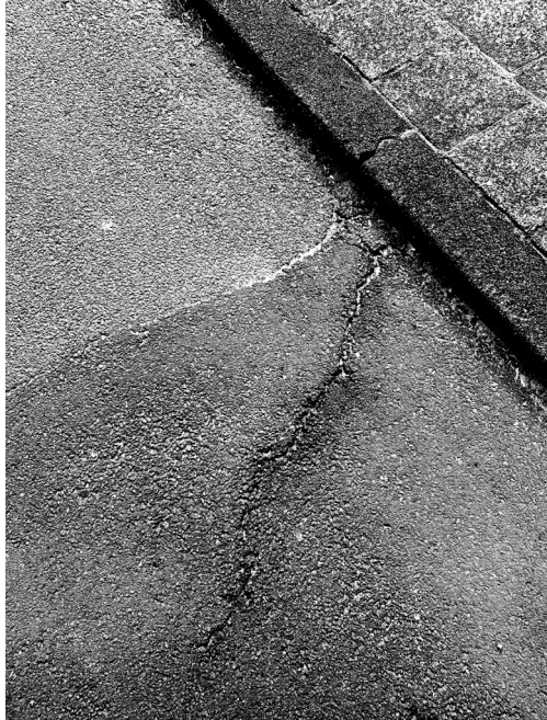
Figure 26: Captured in Rotterdam Noord, 2024: Roots cracking concrete on bike path.
