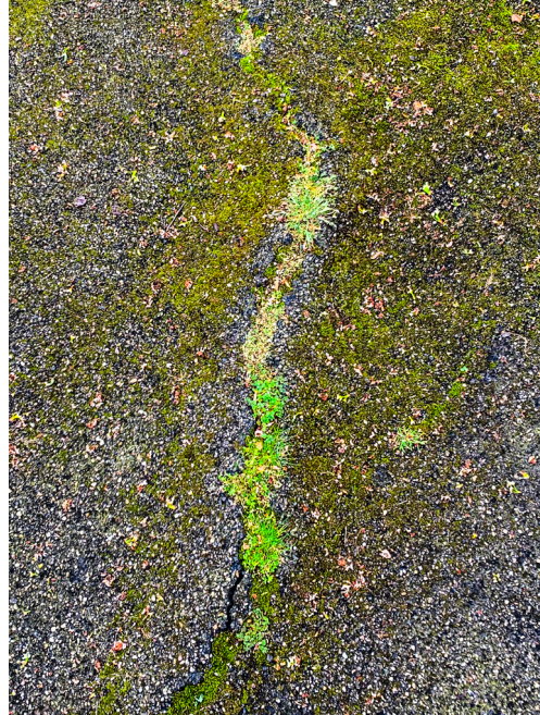
Figure 27: Captured in Rotterdam Noord, 2024: Roots crack concrete with plants growing between.
