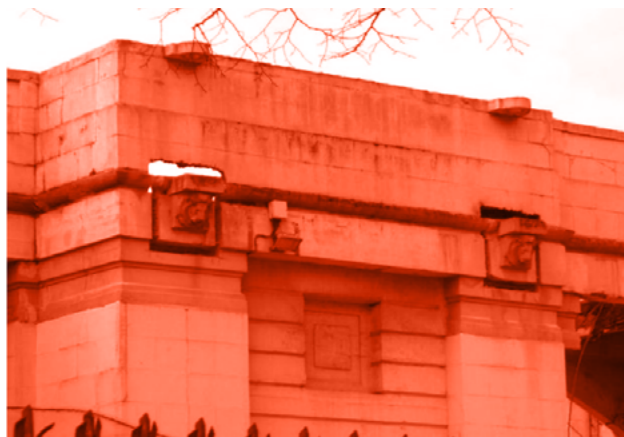
Image 93: Concrete Lion Heads, on the side of the Palace of Industry, in the process of removal for preservation.
