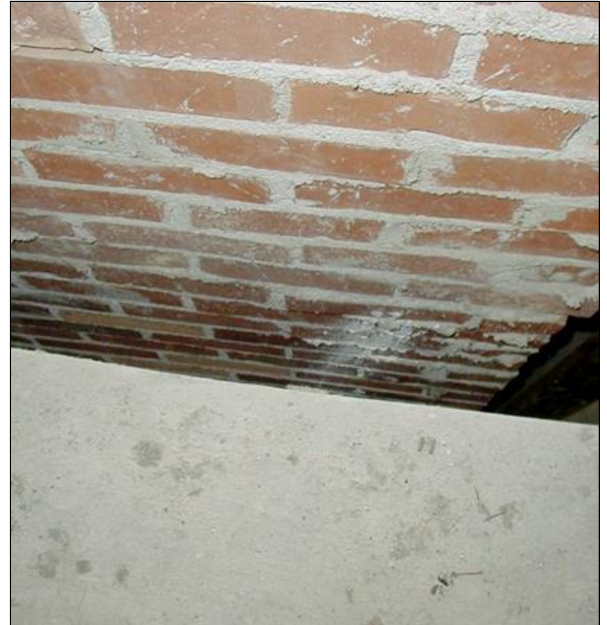
Gaps are left between fireplaces and ceiling framing
