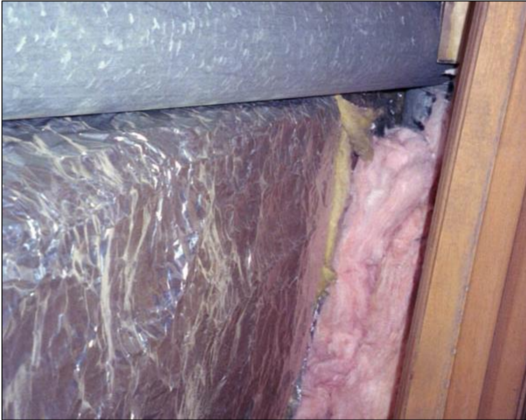
Insulation has been stuffed into the gap in framing between HVAC ductwork and the ceiling framing
