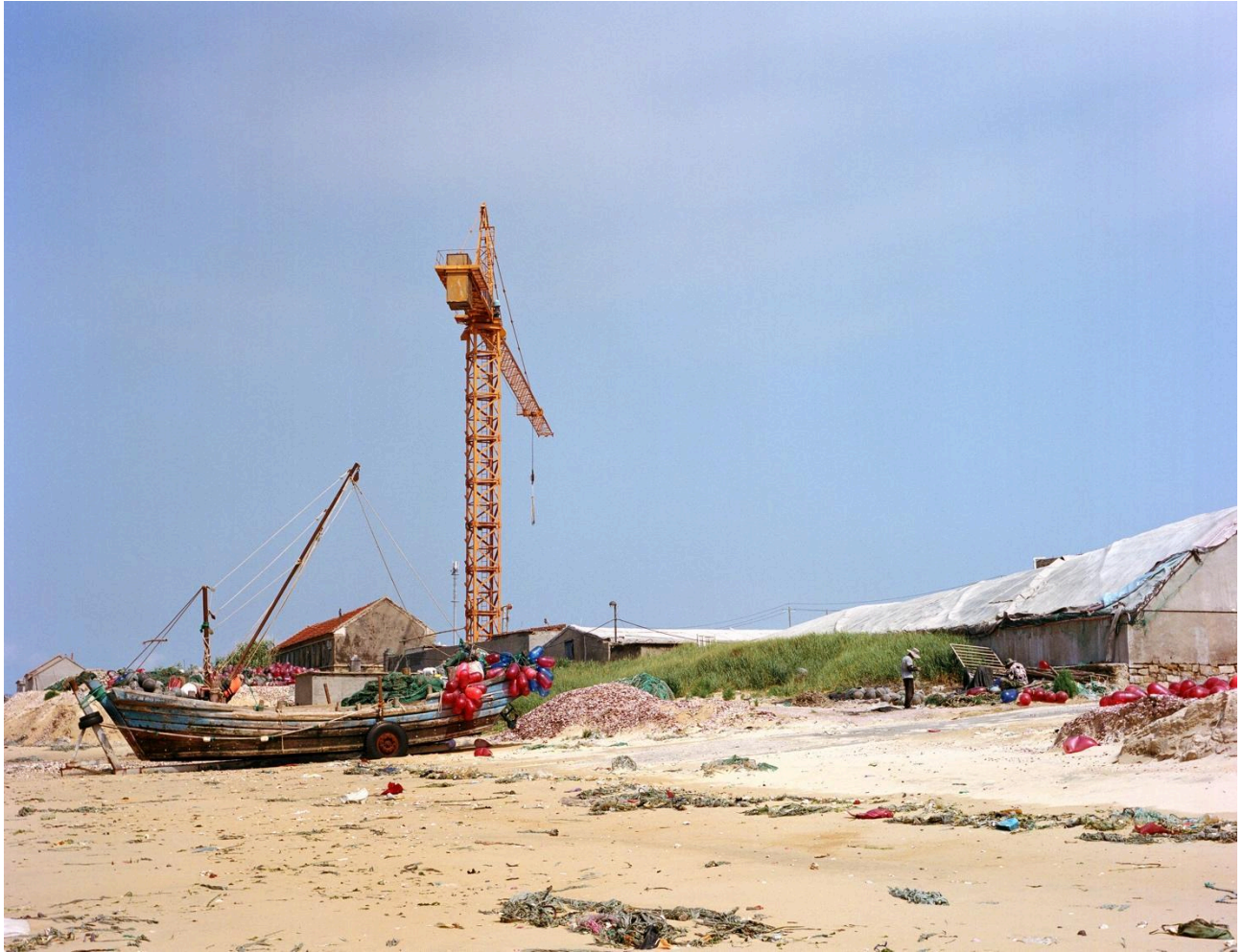
Scallop aquaculture preparations at Jiuguan Town involve loading floats with the help of a tower crane. More than 20 like this are situated along the beach.
