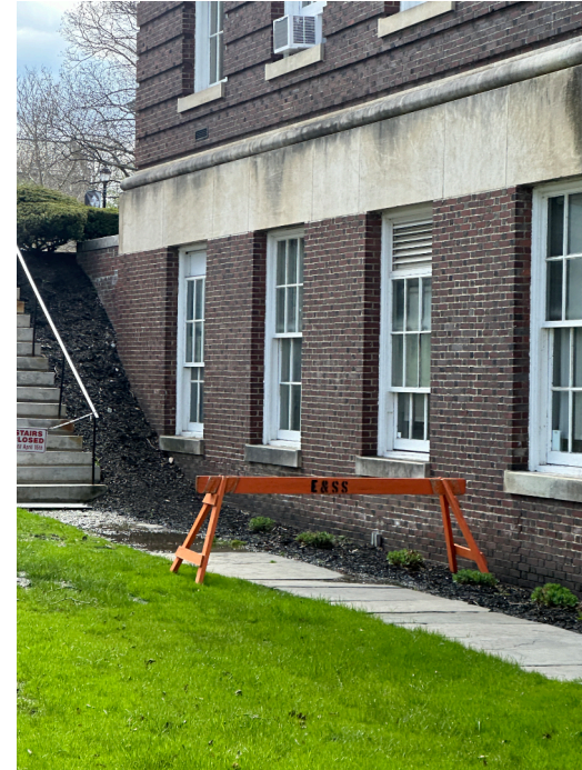
Access to stairs blocked by standing water
