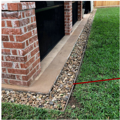
Possible french drain drain cover to line sidewalk filled with matching larger sized crushed stone
