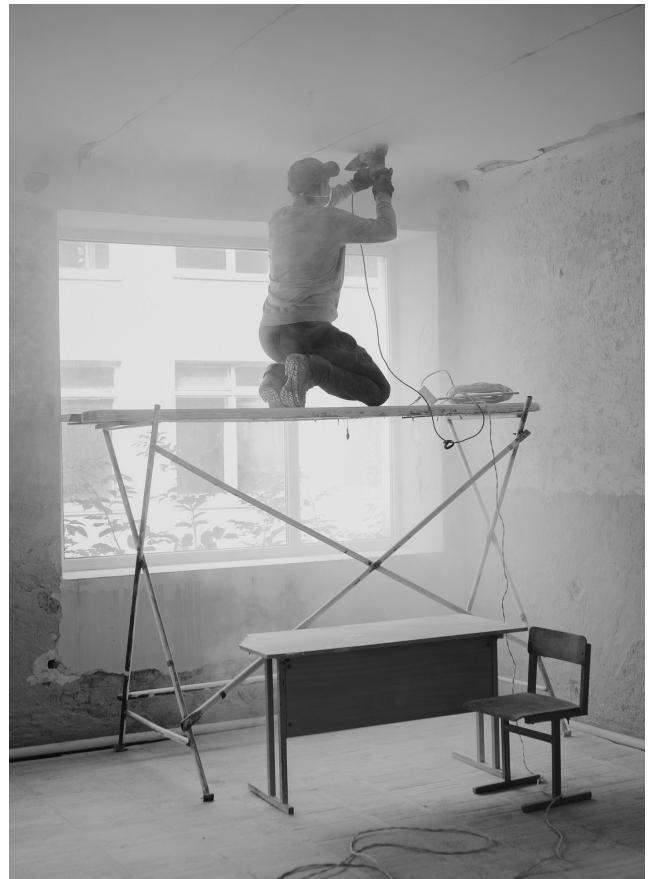
CO-HATY shelter in Ivano-Frankivsk, July 2022. Construction process. Photo: Nastya Kubert (NGO Metalab)
