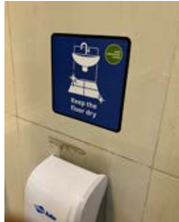
Sticker with faulty hand dryer
