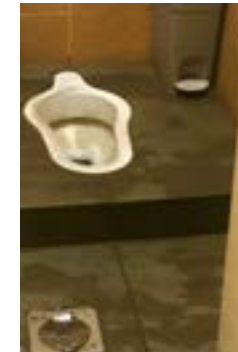
Wet toilet floors
