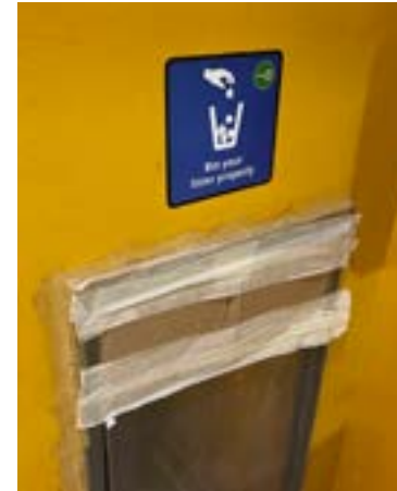
Sticker with unusable rubbish bin
